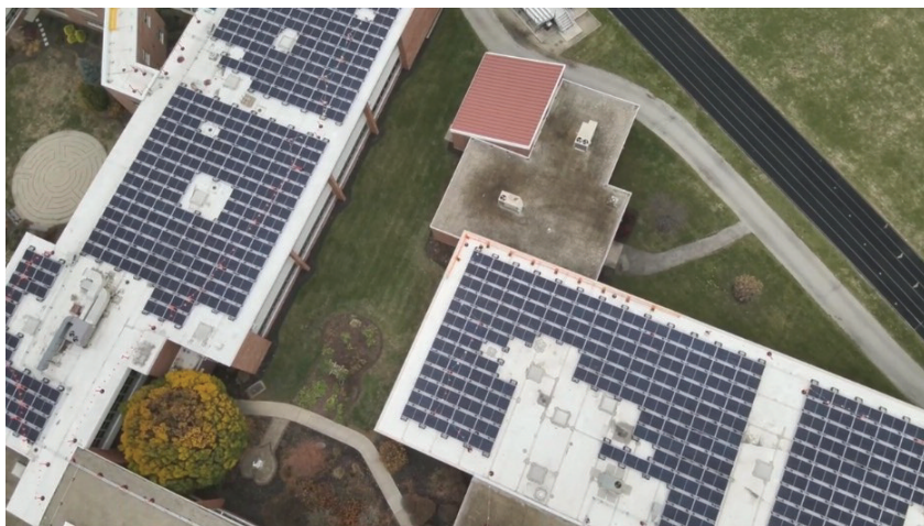
An aerial image of the rooftop solar project at Marist High School in Chicago completed in 2025.
